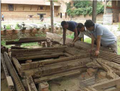
A facade door is being inspected for repairing the Char Narayan Temple.
