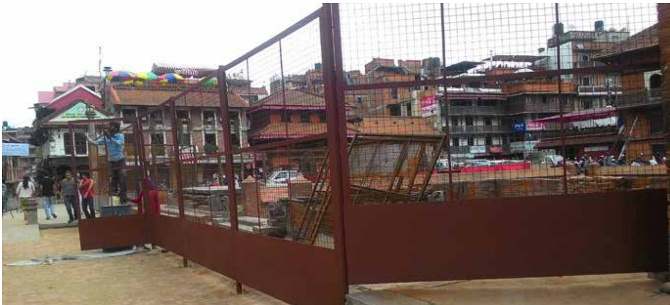
Manimandapa Pati South | June 21, 2016 Building of metal fencing completed around the Pati including red oxide painting.
