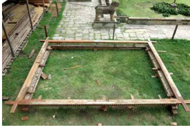
Manimandapa Pati South | May 17 & 20, 2016 The repaired and retrofitted cornices of all four side during and after completely assembled.
