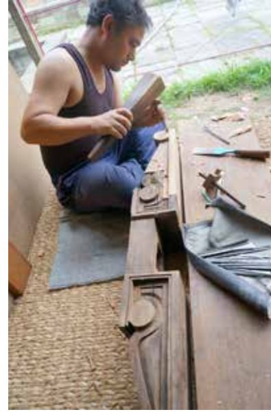
Manimandapa Pati South | May 30, 2016 Repairing, replicating and retrofitting of the central column capital ( meth ) are ongoing.
