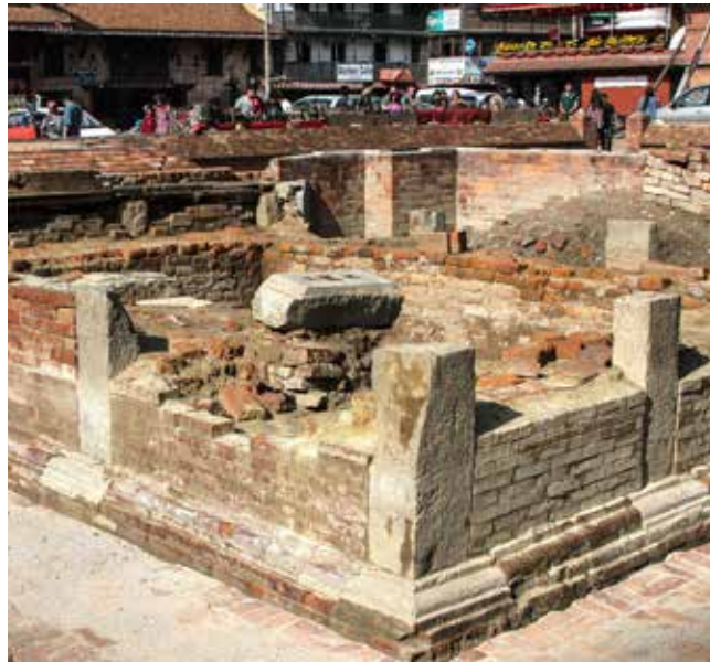
Manimandapa Pati South | May 08 & 12, 2016 Later period brick pavement removed and excavation was carried out around the Pati's plinth to check the condition of foundation where the original brick and stone nagol (bead) were discovered and now it is exposed.
