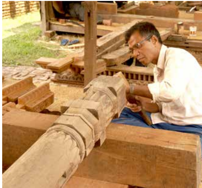
Manimandapa Pati South | May 17 & 20, 2016 Woodcarver Hari Prasad Silpakar replicating the deity as per the original large window's kulan and carpenter repairing the central column.
