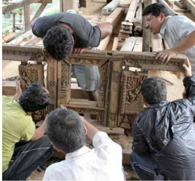
Manimandapa Pati South | May 08, 2016 Carpenters and woodcarvers (Tirtha Ram Silpakar and friends) assembling one of the four large windows after damaged parts were replicated and repaired.
