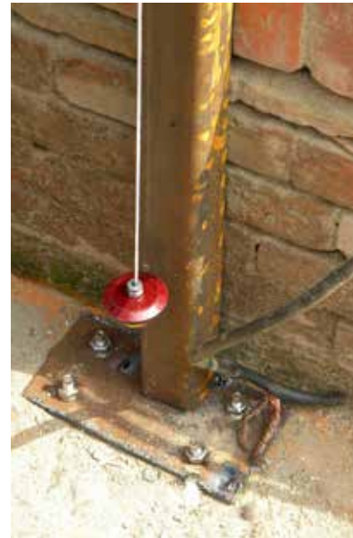
Manimandapa Pati South | June 07, 2016 Metal fencing is being initiated by installing plate on ground erecting square pipe post.
