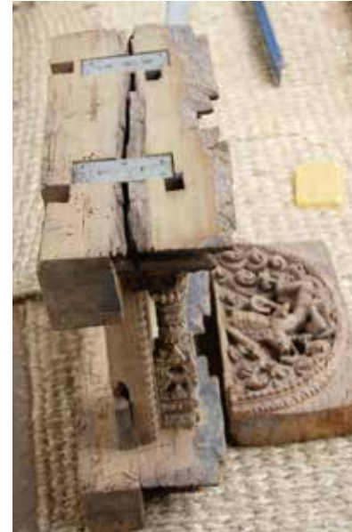
Manimandapa Pati South | May 05, 2016 Broken kulah (cornice) of the window is being joined with the stainless steel plate and screws. Steel plates are used only for joining the completely broken pieces only.
