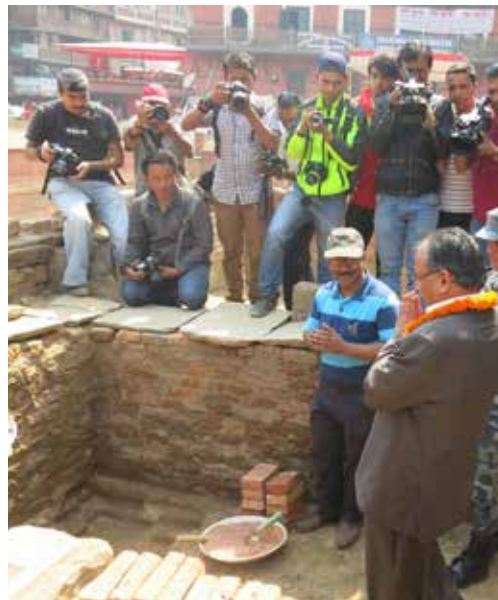
Manimandapa Pati South | April 24 & 25, 2016 Ground floor of the Pati was excavated and trash cleared from site. Former Prime Minister Mr. Puspa Kamal Dahal (Prachanda) inaugurated the rebuilding of Pati by laying foundation brick on northeast corner on April 25, 2016. This inauguration initiated the over all reconstruction of monuments and houses that was destroyed by devastating earthquake of April 25, 2015.
