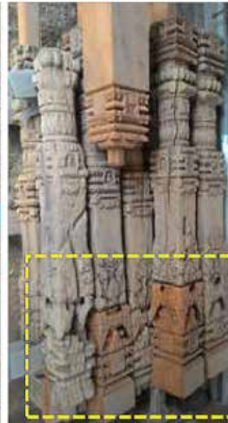
Manimandapa Pati South | March 28, 2016 Carved columns that got deteriorated by time and damaged during the devastating earthquake of April 25, 2015 were replicated, repaired and strengthened for rebuilding the Pati.
