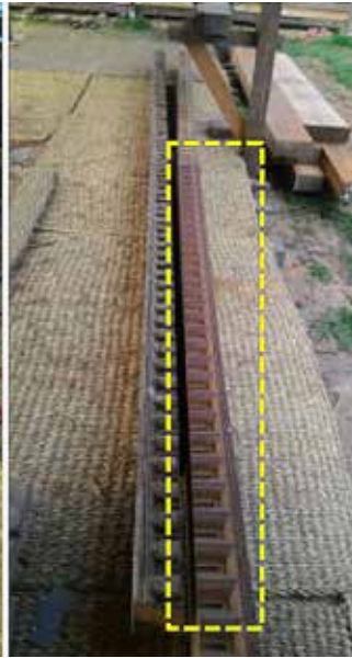
Manimandapa Pati South | March 28, 2016 Parts of cornices that were damaged from April 25, 2015 devastating earthquake were replicated and repaired for rebuilding. Repaired parts are in light color.
